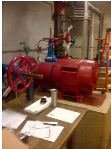
Figure 13. The fire pump assembly.
