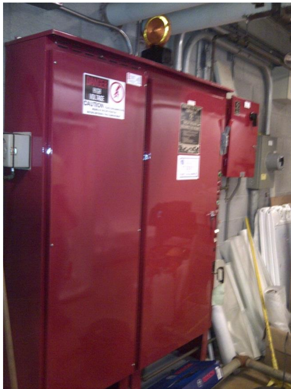
Figure 35. Main fire pump apparatus.
