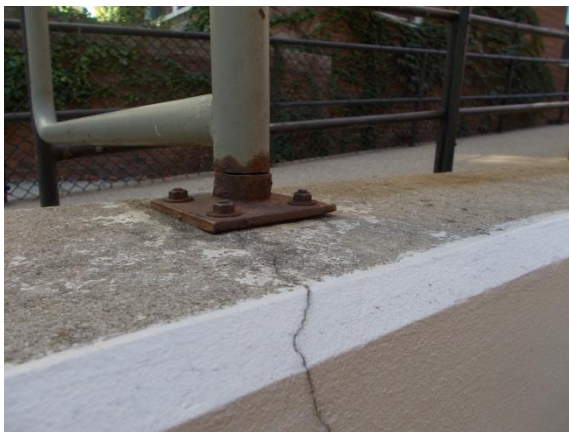
Figure 39. Corrosion of the guardrail and crack in the concrete retaining wall.
