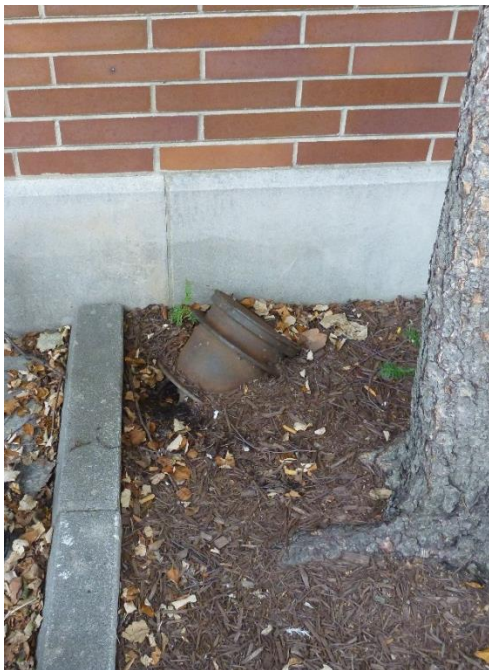
Figure 19. Typical foundation drainage grade cleanout heaved out of the ground.
