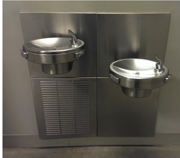
Figure 18. Typical existing electric water cooler.
