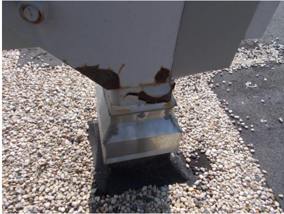
Figure 1. Corrosion on the surface of the structural steel supporting the sound attenuation wall.
