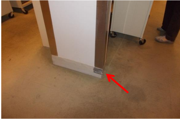
Figure 4. Sheet metal corner guard does not extend to the baseboard. The baseboard in this location has been repaired with duct tape.
