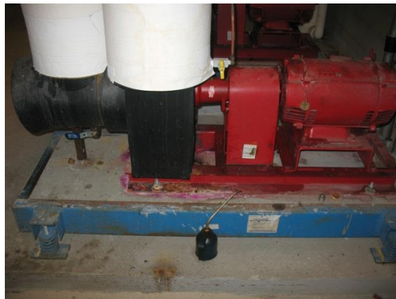
Figure 23. Chilled water pump P-1.
