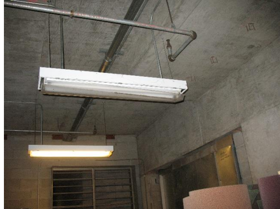
Figure 11. Dry sprinkler piping in mechanical plenum.
