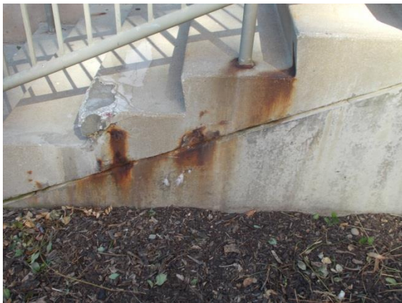
Figure 41. Ferrrous staining on the surface of the concrete at the north stoop.
