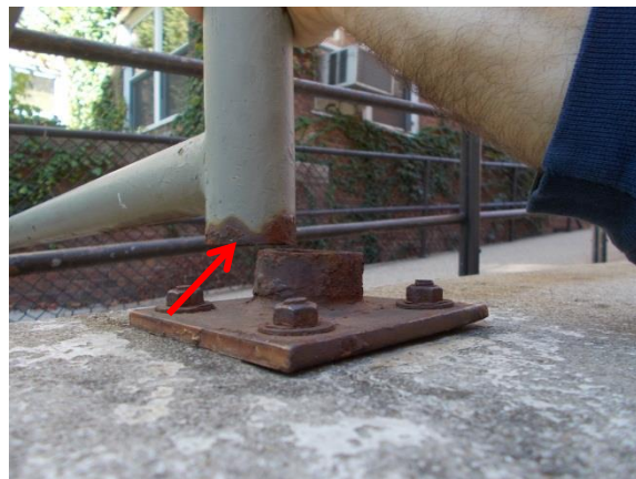
Figure 40. Corrosion related failure of the guardrail connection on the north retaining wall.
