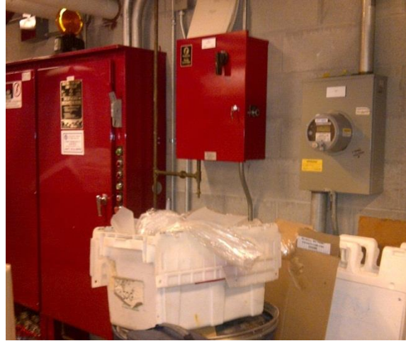
Figure 38. Automatic transfer switch.
