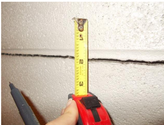
Figure 6. Open crack in the concrete masonry wall between the fourth floor mechanical and air handling rooms.
