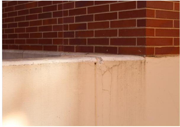
Figure 44. Crack in a north side retaining wall.
