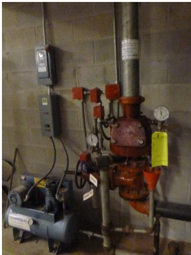
Figure 12. Dry valve and compressor serving fourth floor dry system.
