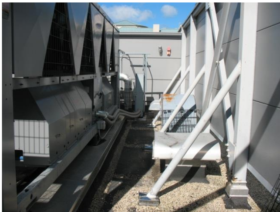
Figure 22. Air cooled chiller.
