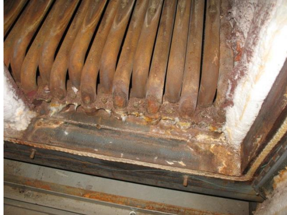
Figure 21. Corrosion on fire side of boiler tubes.
