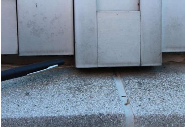
Figure 3. A window mullion on the east facade that has shifted downward.
