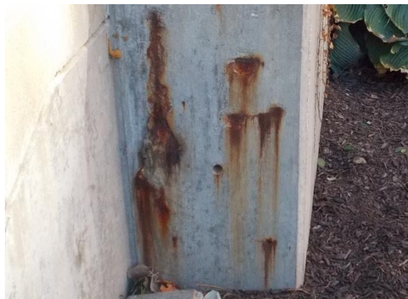
Figure 42. Ferrrous staining on the surface of the concrete at the north stoop.
