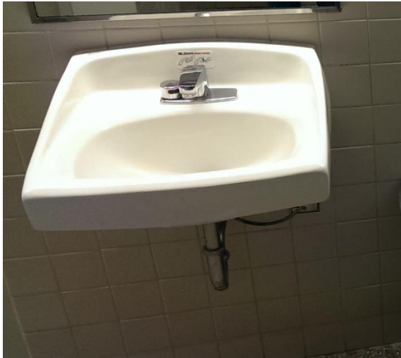
Figure 17. Typical wall hung lavatory with sensor operated faucet.
