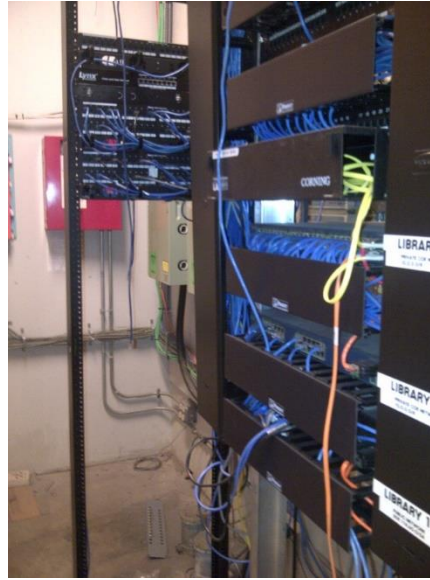
Figure 29. Single rack in IT Room.
