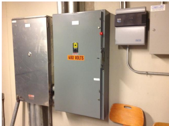
Figure 26. Square-D motor control center.
