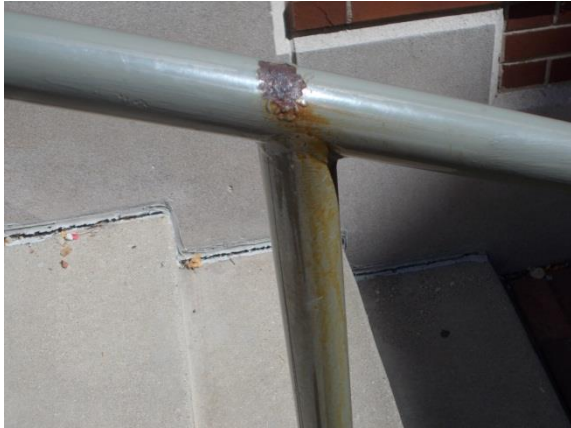
Figure 43. Typical handrail surface corrosion.
