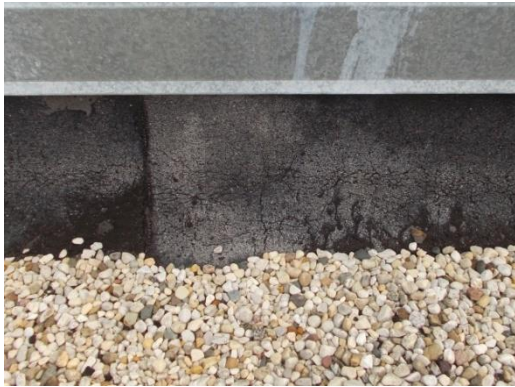
Figure 2. Cracking on the surface of the upturned roofing
