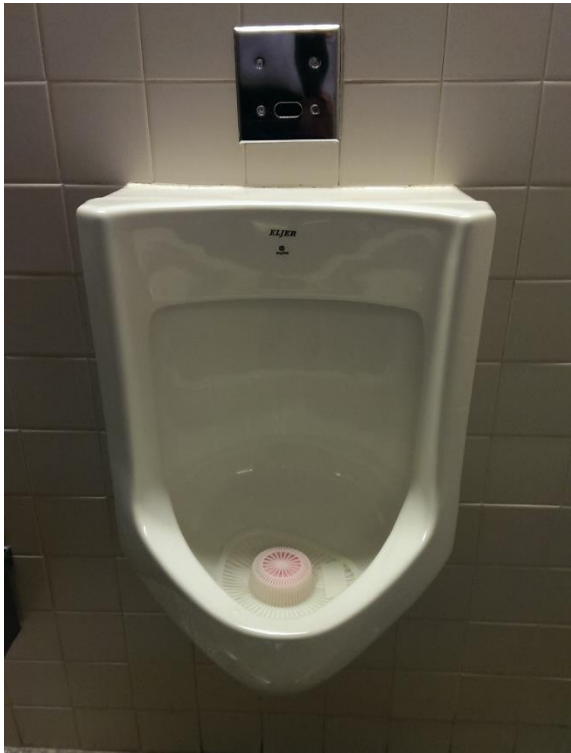
Figure 15. Typical wall hung urinal with concealed sensor operated flush valve.
