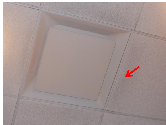
Figure 7. Dirt present on tile adjacent to a ceiling vent.
