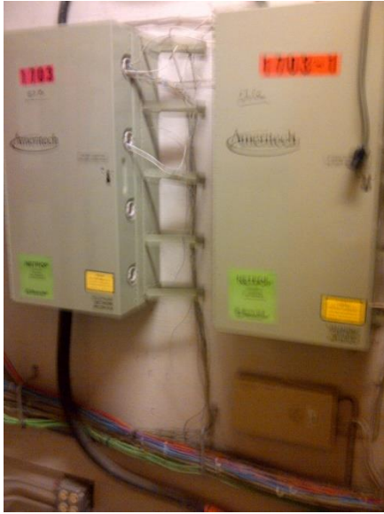
Figure 28. Ameritech telephone equipment found in IT Room.
