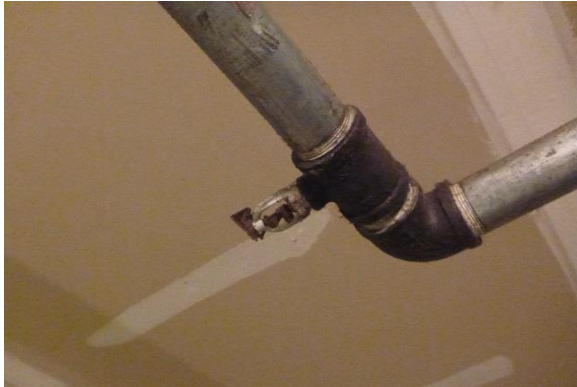
Figure 14. Side outlet sprinkler head in mechanical space.
