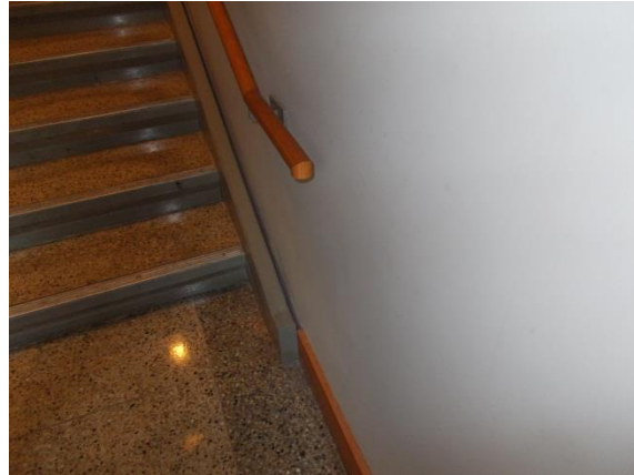
Figure 9. Existing hand rail extends beyond the bottom riser and stops abruptly. The 2010 ADA standards require that the handrail return horizontally to the wall surface at right.
