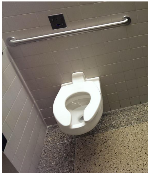
Figure 16. Typical wall hung toilet with concealed sensor operated flush valve.
