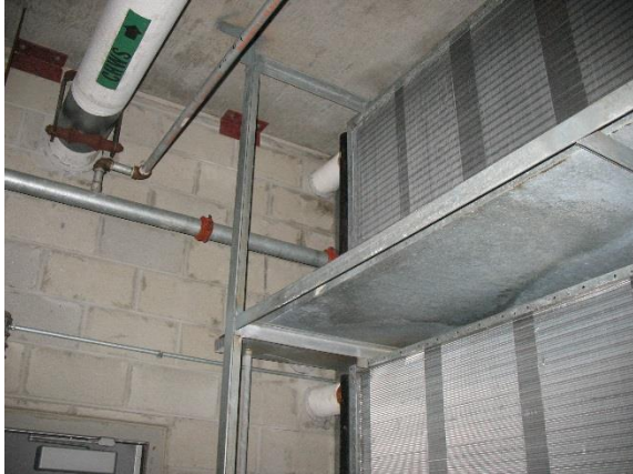
Figure 10. Dry sprinkler piping in mechanical plenum.
